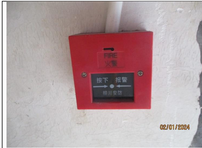
Fire alarm button
