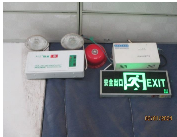
Exit sign, emergency light and fire alarm
